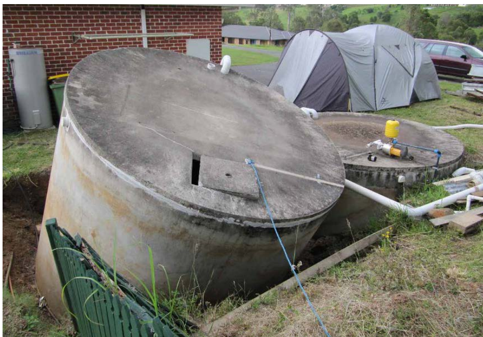
Water tanks in waterlogged ground can be a big problem
